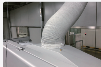
Exhaust Hood and Pipe
